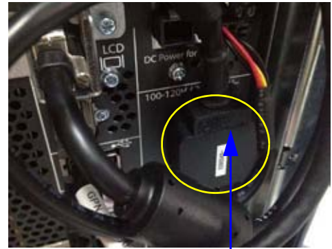
Printer Power cable in Nest box
